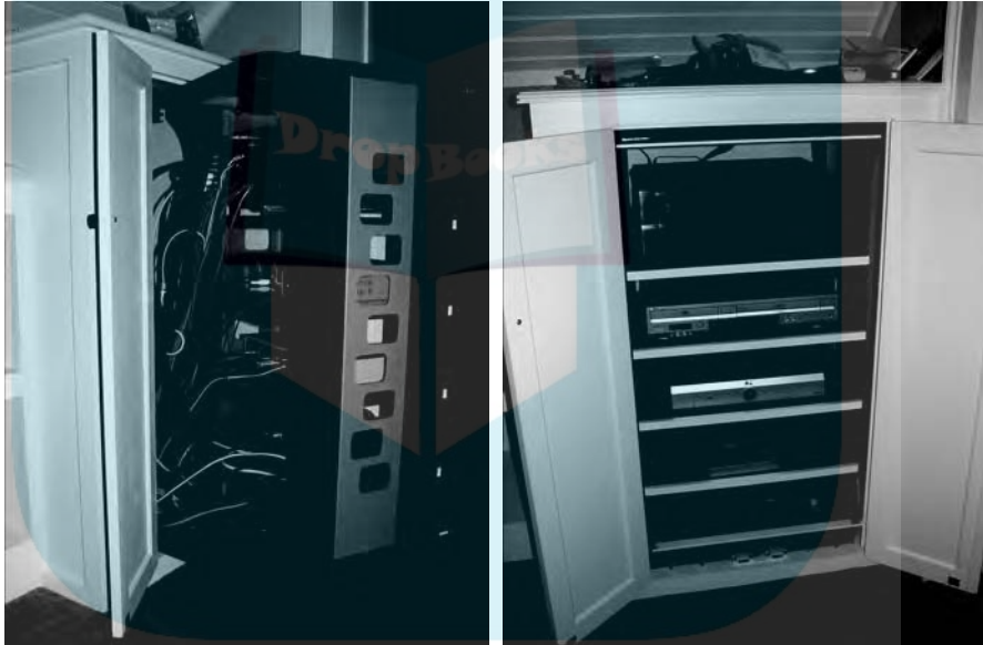
Figure 2-3: Danny's rack allows access to his back panels without disconnecting wires.
